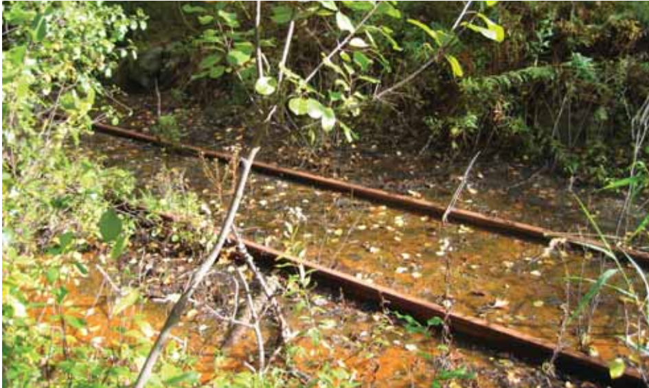
Overgrown vegetation and poor drainage are typical conditions of the rail corridor behind the Miracle Mile.
