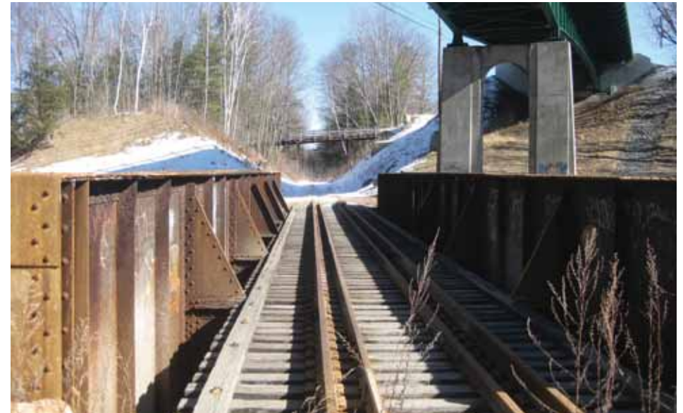
Above, rail bridge above the Mascoma River, and below Route 4. The wooden overcrossing is in the distance.
