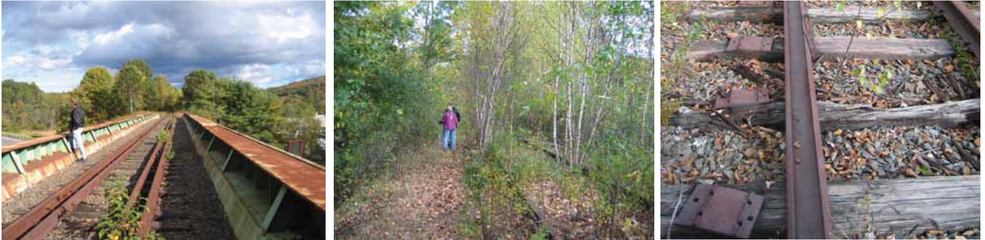
Scenes from the Central Segment of the corridor: Left, I-89 bridge crossing; center, overgrown vegetation typical of this segment; right, dismantled train tracks.
